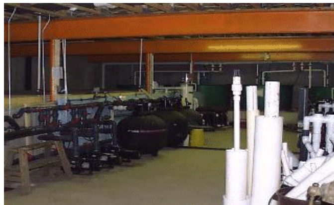
Holding tanks, filters, coolers, and UV light system
